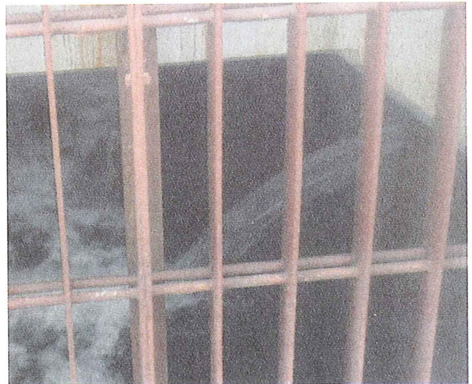
Leak from trench wall flowing into breakwater lagoon
